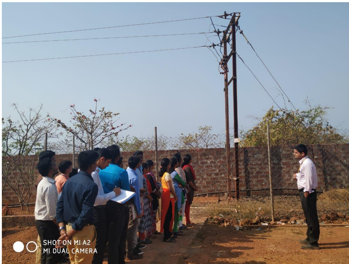
Near 11kV incomer 2 pole structure
